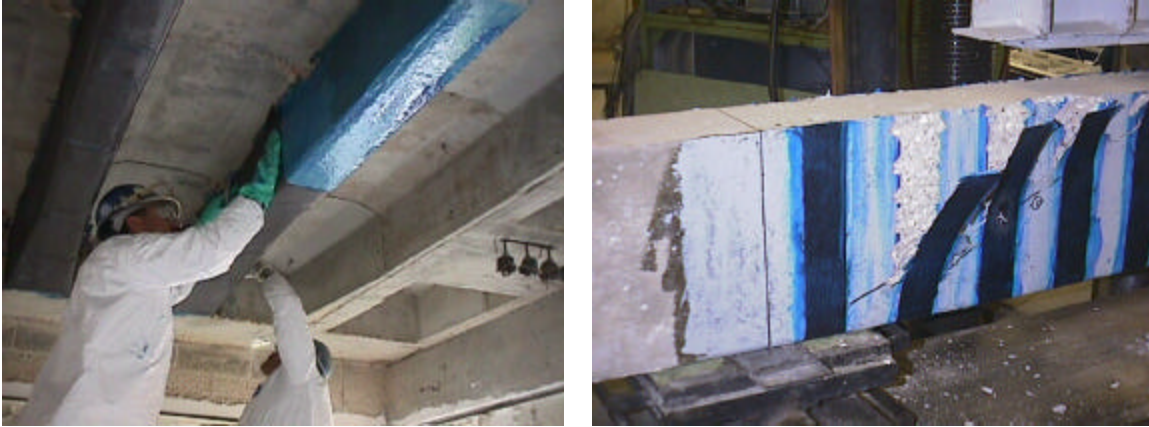
Figure 1, left: Application of FRP sheet on one-way joist. Figure 2, right: De-lamination of externally bonded FRP sheets.
