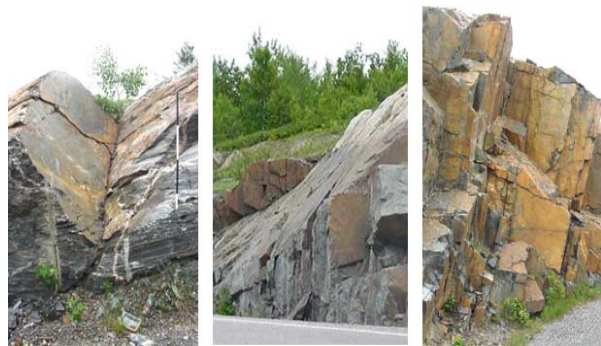
Figure 1: (left) Example of wedge, (middle) planar, and (right) toppling failures along road cuts.
