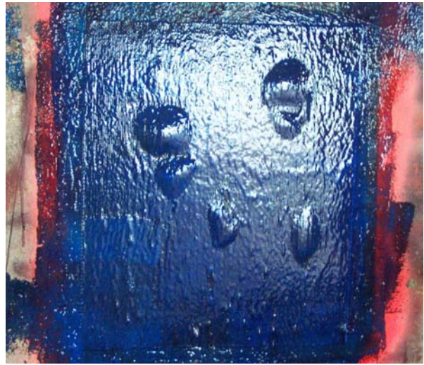
Figure 13: "Forced" delamination by air injection.
