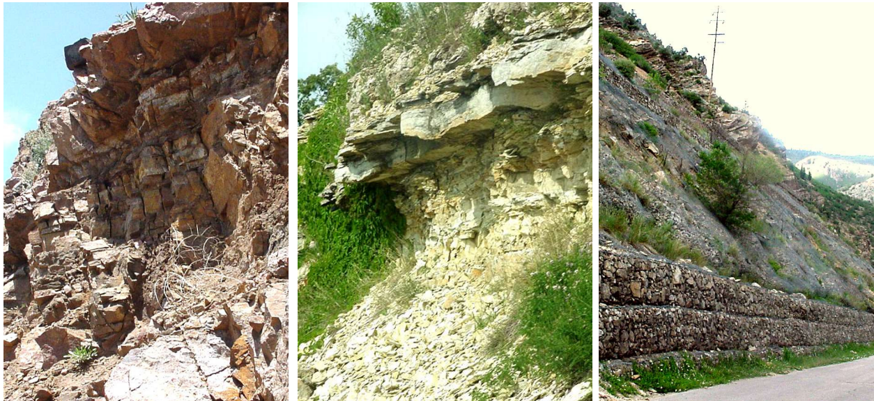
Figure 6. Example of raveling, undercutting, and rolling failures along road cuts.
