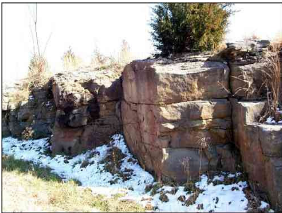
Figure 2: Orthogonal nature of joint sets. Measurements of the “cracks” or discontinuities are displayed in Figure 3.
