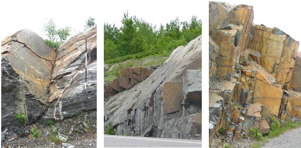
Figure 1. Example of wedge, planar, and toppling failures along road cuts.
