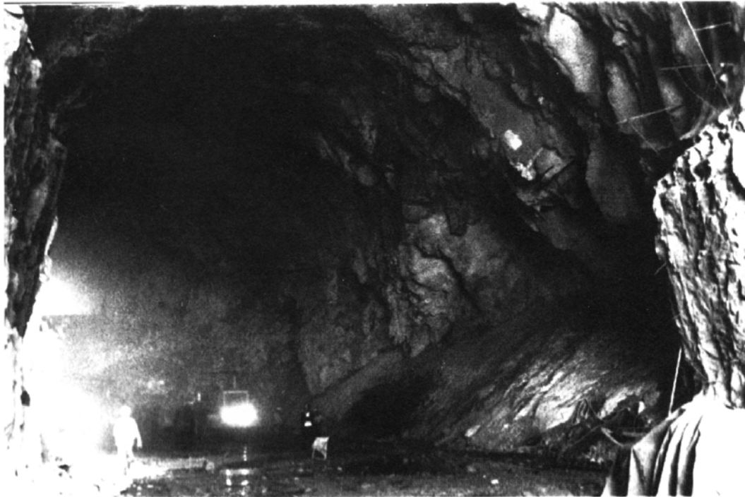
Fig. 1. Massive overbreak in the Aquamilpa diversion tunnel
