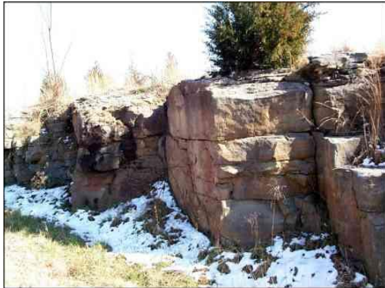
Figure 1.2: Orthogonal nature of joint sets. Measurements of the “cracks” or discontinuities are displayed in Figure 1.3
