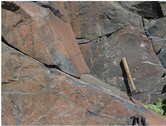
Figure 1. A rock mass showing a discontinuity along which a rock block slid. The block at the top left corner is also likely to slide with time.
