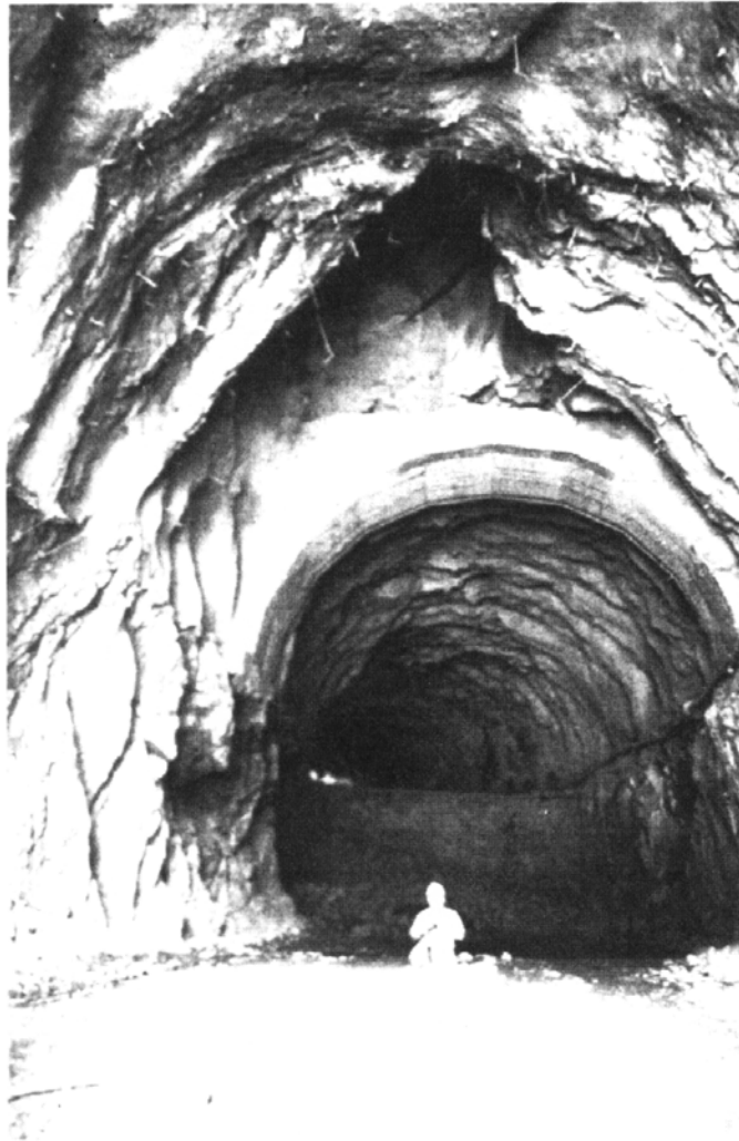
Fig. 1. An example of massive overbreak in the Aqua Milpa tunnel, Mexico
