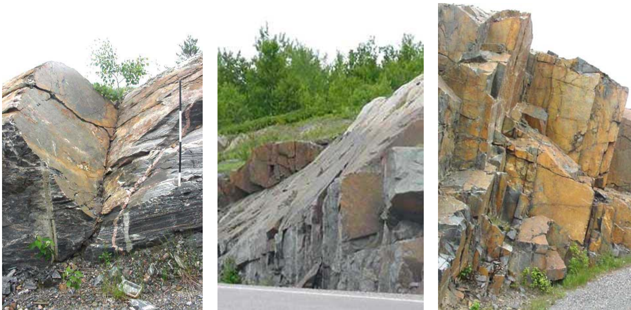
Figure 4. Example of wedge, planar, and toppling failures along road cuts, respectively, Sudbury, Canada.
