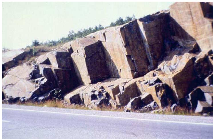
Figure 2. The discontinuous nature of rock masses (Highway cut in Nova Scotia, Canada)
