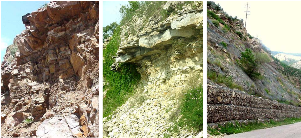
Figure 3. Raveling, undercutting, and rolling failures along road cuts, respectively, Colorado, Highway 70.
