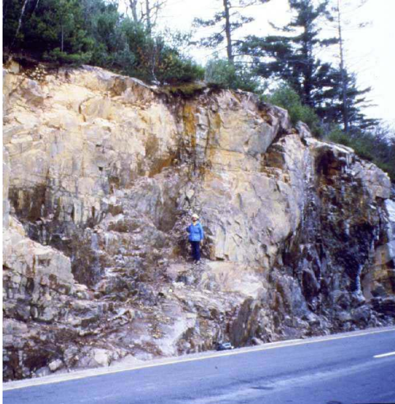
Figure 5. Failed rock cut, Hwy 401, Brockville, Ontario, Canada, after removal of rubble. The failed material released along a sub-vertical joint, exceeded the capacity of the ditch, spilled out onto the left lane to a depth of one meter, resulting in the death of a truck driver.
