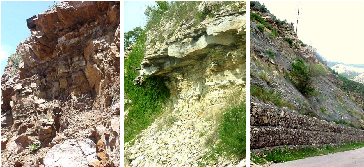
Figure 4. Raveling, undercutting, and rolling failures along road cuts.
