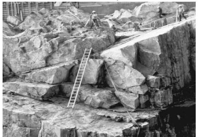
Figure 1. Powerhouse excavation in northern Manitoba, Canada, showing discontinuity controlled failures in granitic gneiss.
